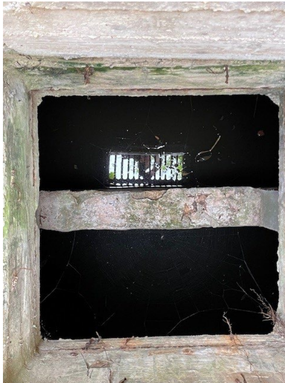
CS #1 - IN-LINE WEIR in INLET STRUCTURE
