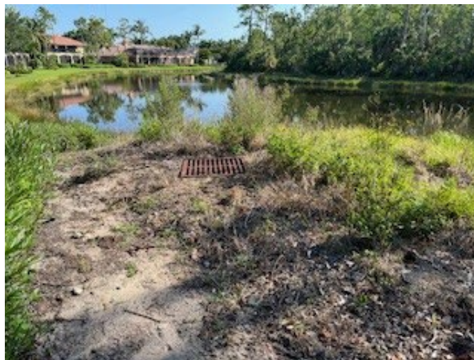
CS #2 - INLET STRUCTURE with IN-LINE WEIR
