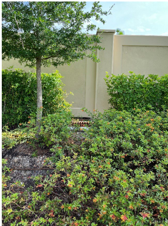
CS #1 - INLET STRUCTURE with IN-LINE WEIR
