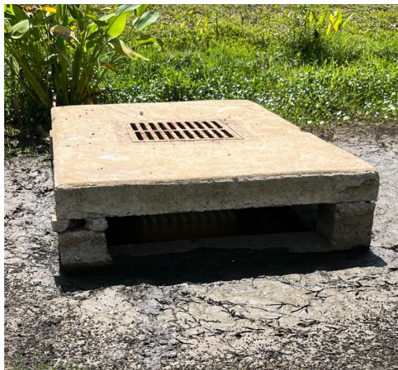
BUBBLE UP STRUCTURE IN IGE PERIMETER DITCH
